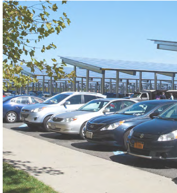
example of a parking lot solar canopy (photo: Blue Oak Energy)
